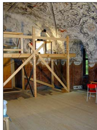
Figure 1: From the 2001 conservation campaign at the west wall. Note the preliminary wooden floor – a measure undertaken in order to check its buffering capacity on the indoor climate
