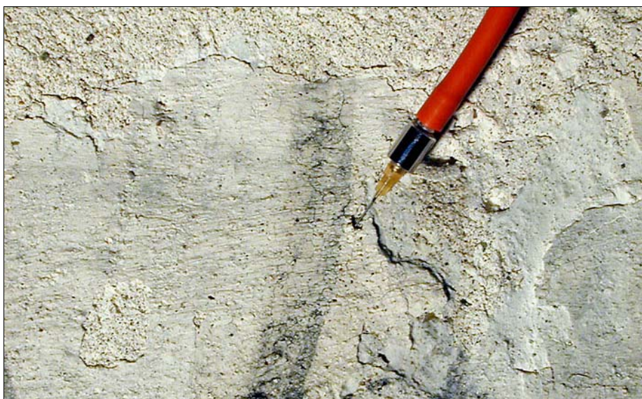
Figure 10: Applying drops of limewater over a longer period of time with an injection needle in order to moisten the plaster before application of consolidants.
