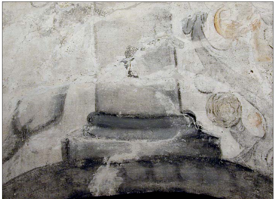
Figure 6: After removal of gypsum from 1966 and application of lime mortar repairs just above the west door
