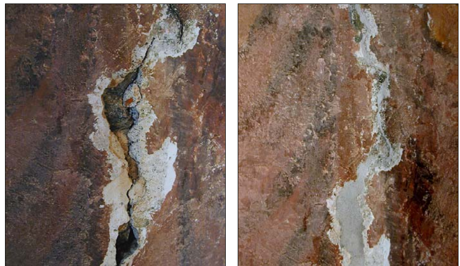
Figure 7: After removal of gypsum from 1966 and application of lime mortar repairs in a crack on the south side
