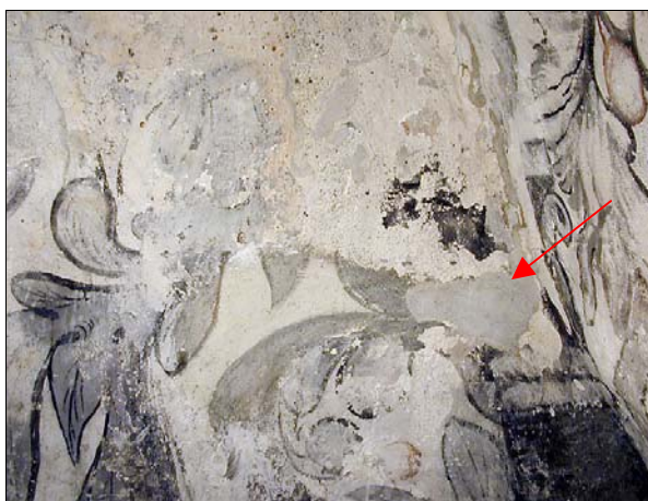
Figure 4: Same area as in fig.3 after application of new lime mortar
