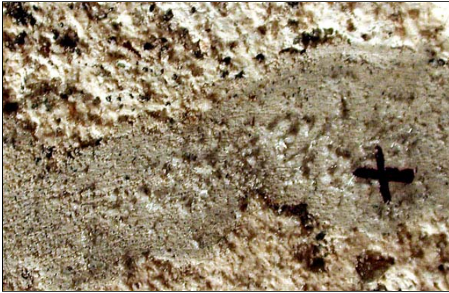
Figure 26: Salt whiskers on a new lime mortar repair. Salt has a tendency to effloresce on such material because of its finer pores, which keeps moisture longer, as compared to the adjacent old lime plaster. The area was not sampled in order to be able to follow the evolution of the whiskers in the future. Width of photo c. 5 cm. Photo no. RE02_002.
