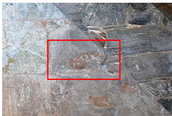
27.1.2020: Over 80% RH, fuktig
